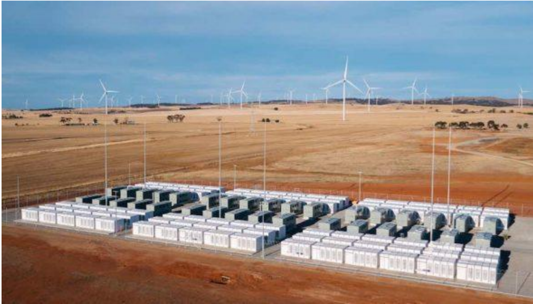
Hornsdale Power Reserve Tesla's "BFB" , opened December 2018
