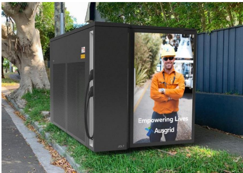
Ausgrid/Jolt EV charging powerbox.
