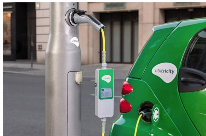
Ubitricity light-pole EVSE in use. Image: Ubitricity
